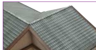
Grime-Stained Roof Detail
